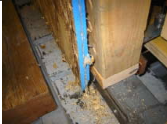
Figure B1. Typical controlling failure mode. Slots shown in lumber end post from nails working (note: slots oriented toward panel centroid). Wall 7.
